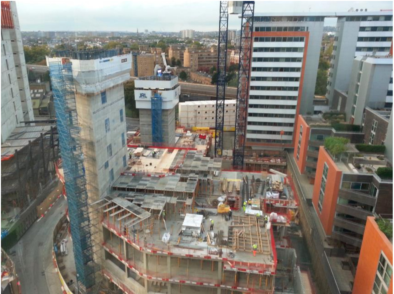
View of site from North Wharf Road in October 2017 (works have progressed significantly since).
